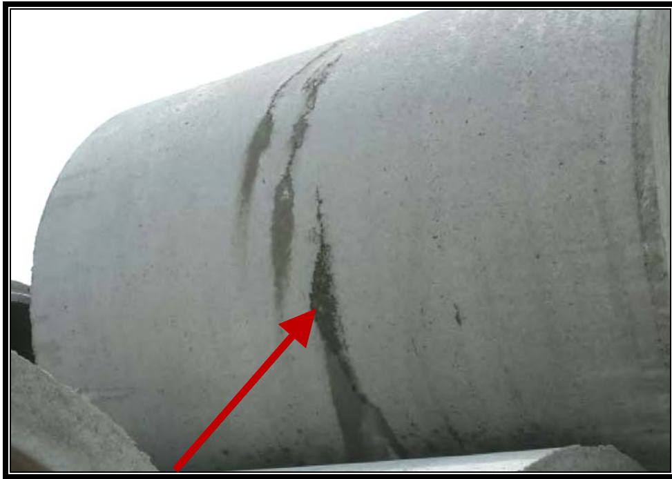
Figure 5-3. Crack Exceeding 0.01 in. and 12 in. in Length – Not Acceptable
