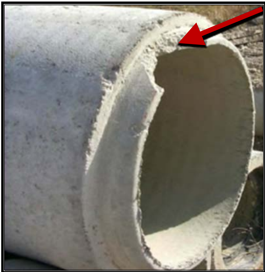
Figure 2-5. Chipped Spigot End – Repairable
