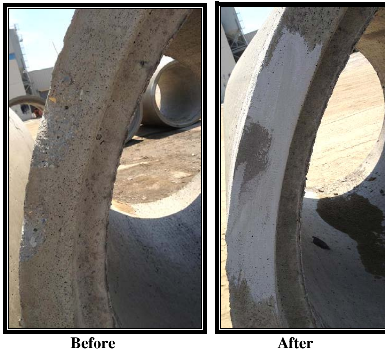
Figure 2-13. Bell Chip Repair - Acceptable
