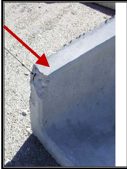
Figure 2-6. Damaged Flared End Section – Repairable.
