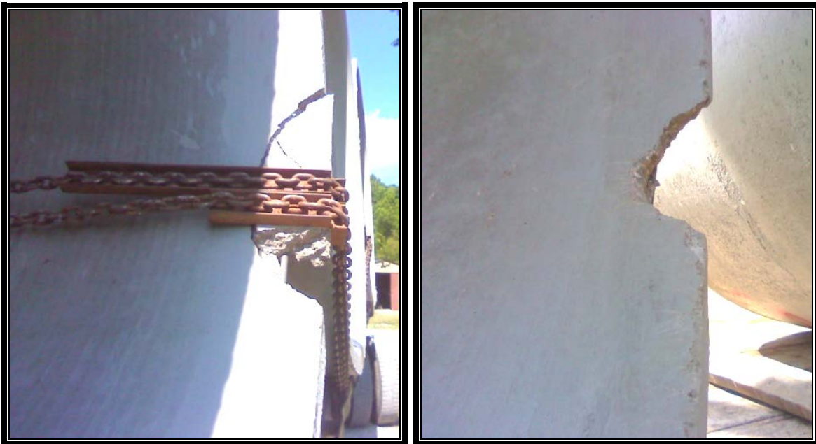
Figure 2-7. Shipping and Handling Damage – Repairable
