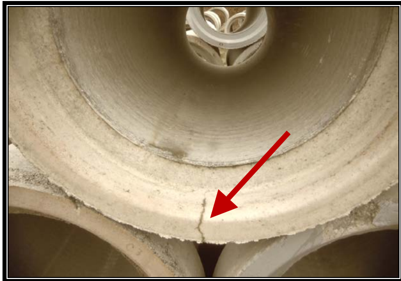
Figure 2-16. Single End Crack – Acceptable
