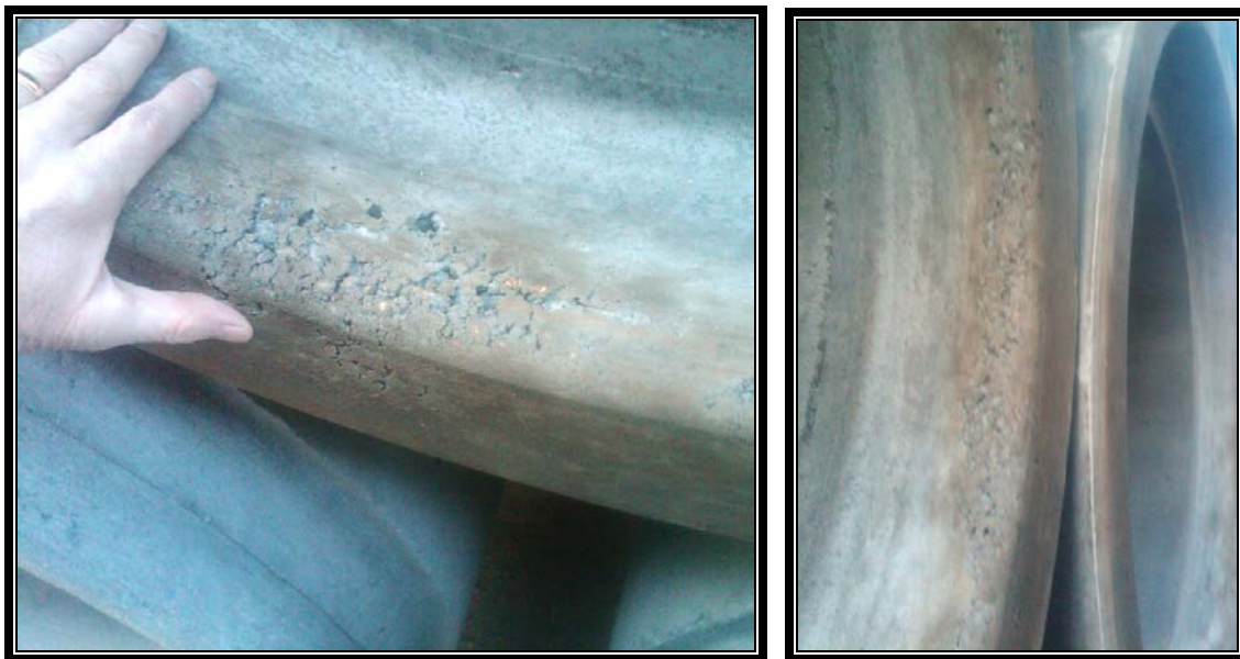
Figure 2-9. Bell Surface Roughness - Acceptable
