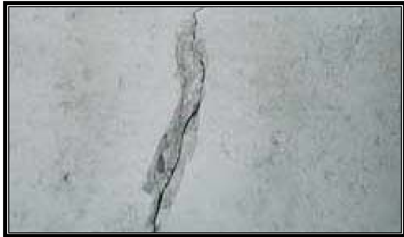
Figure 6-13. Spalling Along Edge of Crack
