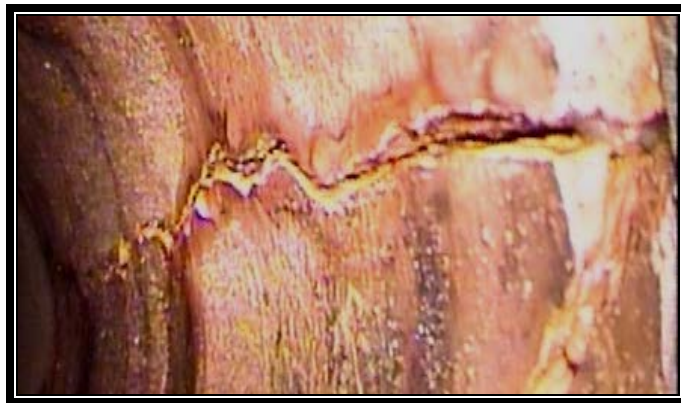
Figure 6-8. Longitudinal Crack > 0.10 in. (courtesy of NASSCO)
