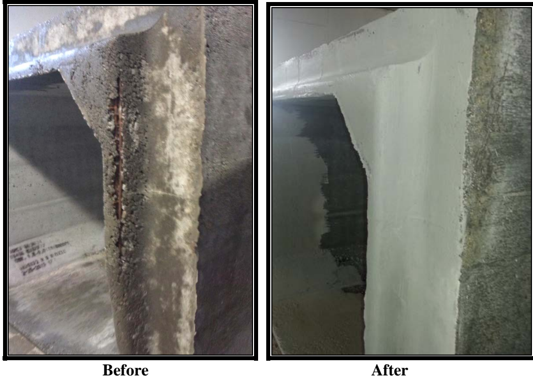
Figure 2-12. Box Culvert Spigot Repair - Acceptable
