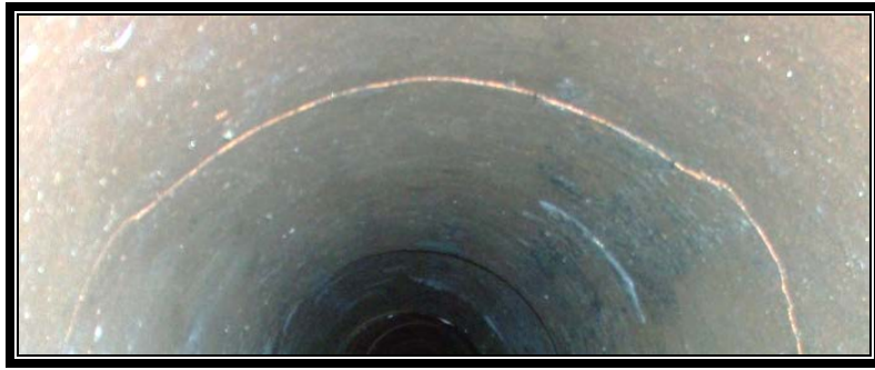
Figure 6-12. Transverse Crack (courtesy of NASSCO)
