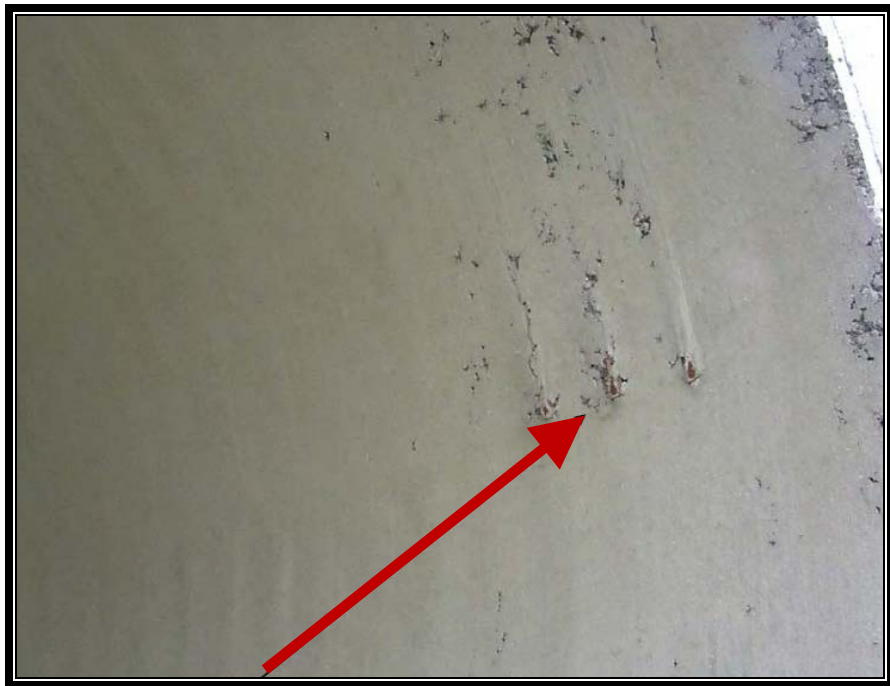
Figure 4-4. Exposed Pipe Reinforcement – Not Acceptable
