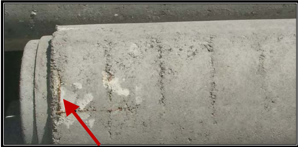
Figure 4-3. Exposed Pipe Reinforcement – Not Acceptable
