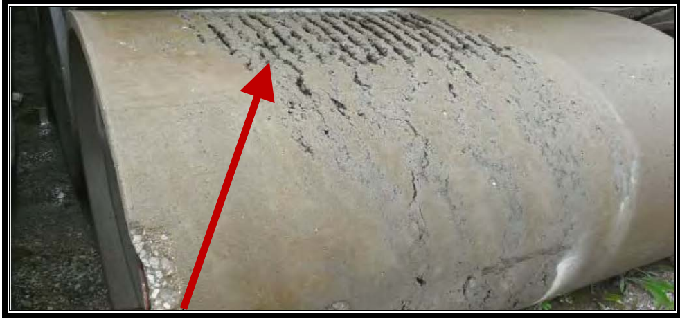
Figure 4-7. Exposed Elliptical Pipe Reinforcement – Not Acceptable
