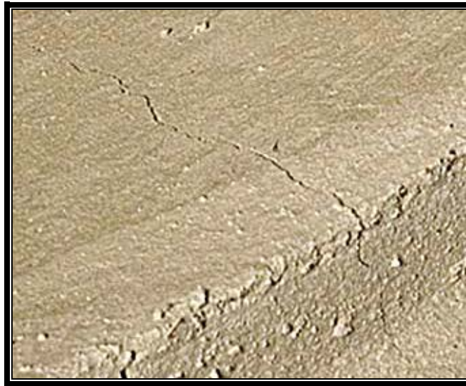
Figure 6-3. 0.01 in. Crack Obtained by Video Inspection
