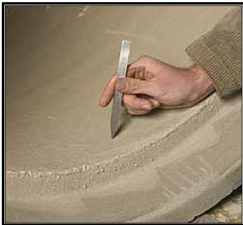
Figure 6-1. Measuring Crack with Leaf Gauge
