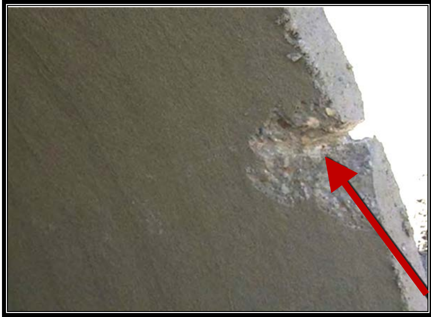
Figure 2-4. Chipped Spigot End – Repairable
